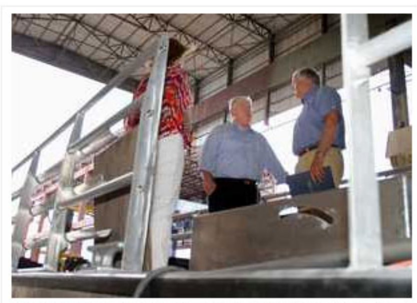
TIM ISBELL/SUN HERALD Gov. Haley Barbour talks with Trinity Offshore President John Dane aboard an oil-skimming boat under construction in Gulfport on Tuesday afternoon.
